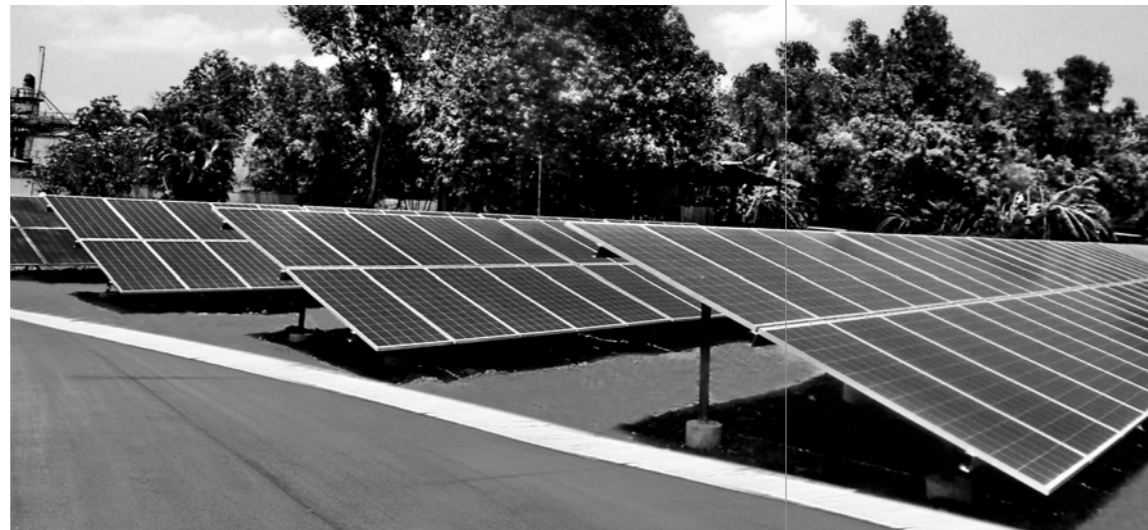
Solar panel installation at Roha plant reduction of CO 2 footprint through solar power generation
